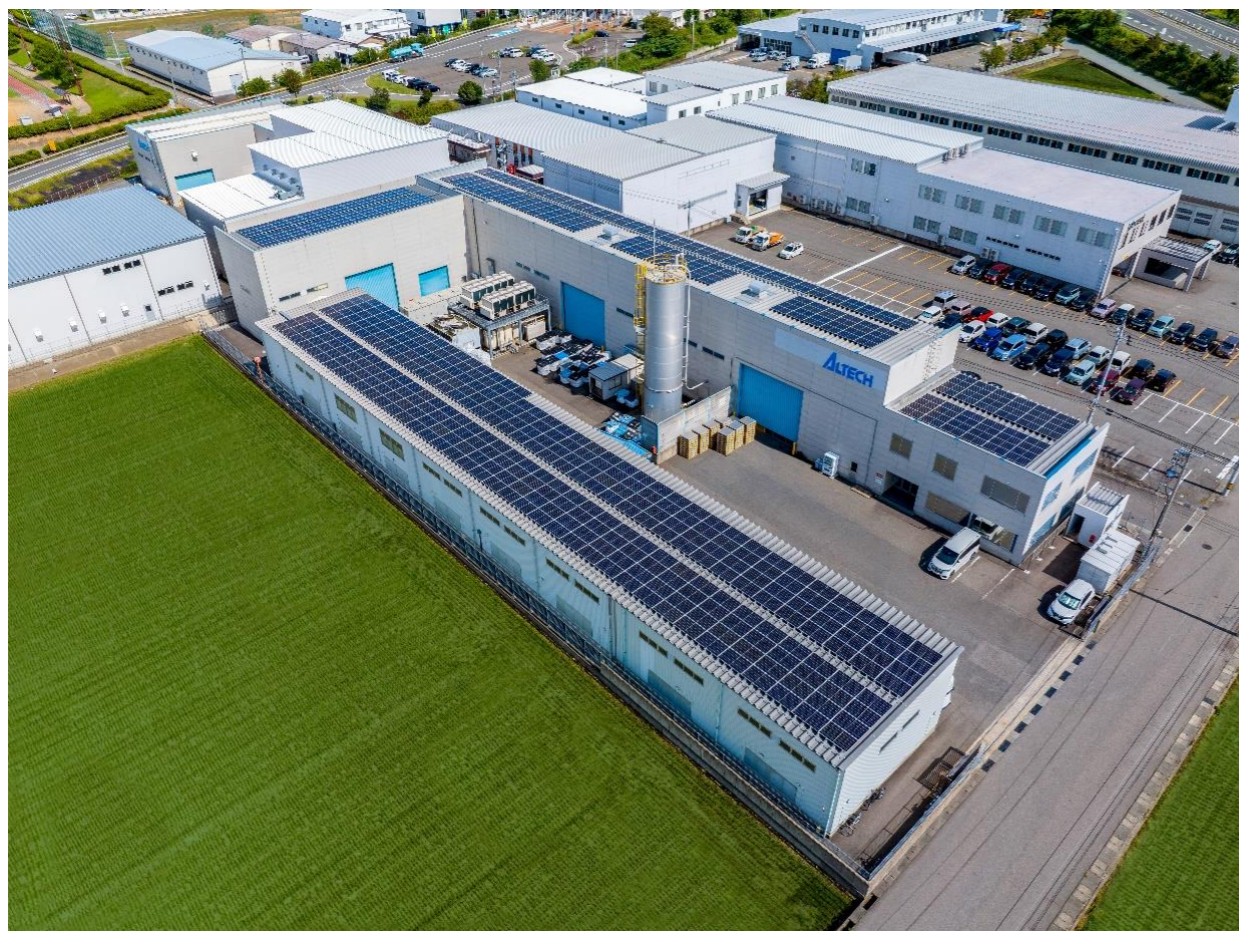
Solar power generation equipment of the roof of Altech New Materials (Fukui) plant
